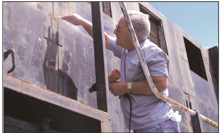
John Ivansco uses a heat gun to enable the painted-over Penn Central letters to be scraped off. In addition to helping with this restoration, he has helped in the yard in a number of ways.
