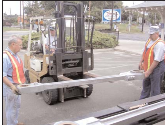
Volunteers Bill Britt and Glenn Miller support one of the rods while the forklift lifts it.
