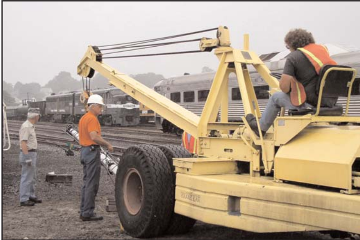
Ira Pollack operating the crane, which will raise the semaphore into position. Dave Roberts at left and Bruce Van Wyk center.
